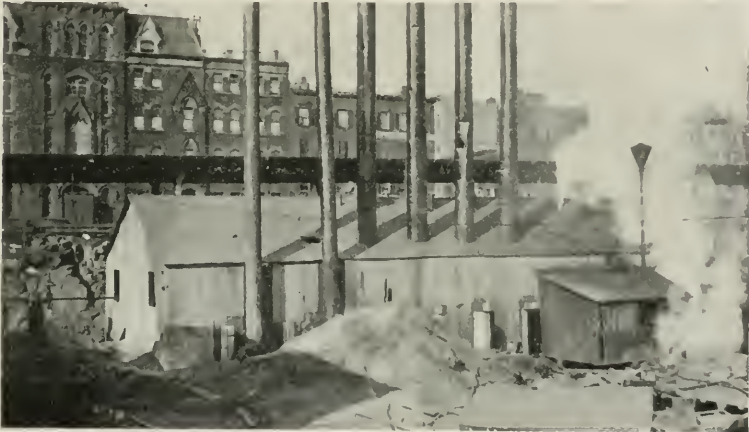
FIG. 1.—Temporary Power House, Pennsylvania Terminal.
